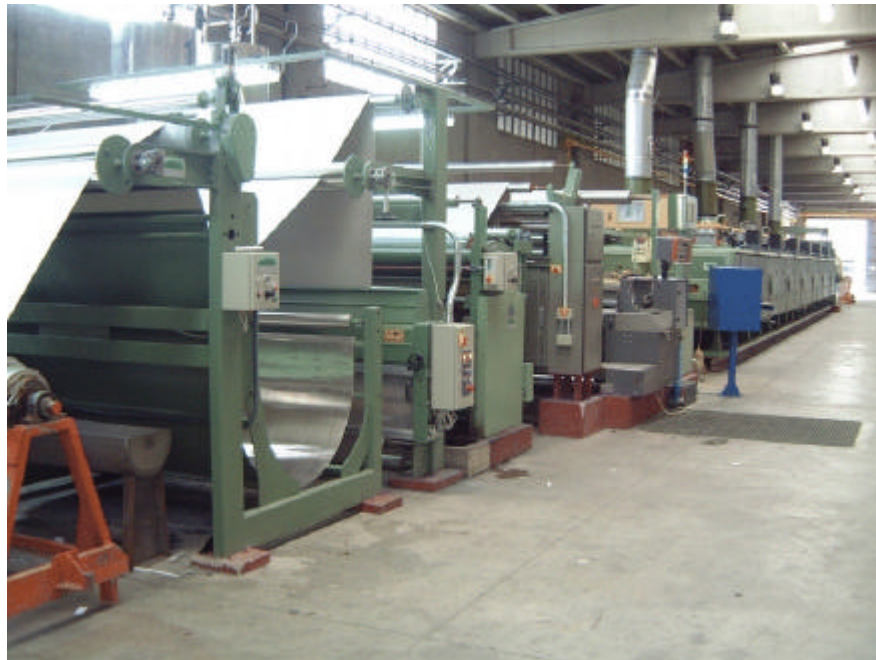
Drying and thermosetting unit 7 chambers
