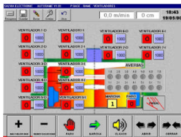
Chamber's blowers control screen
