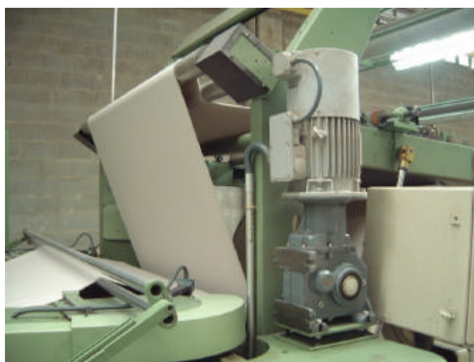
Winding system by charge cell
